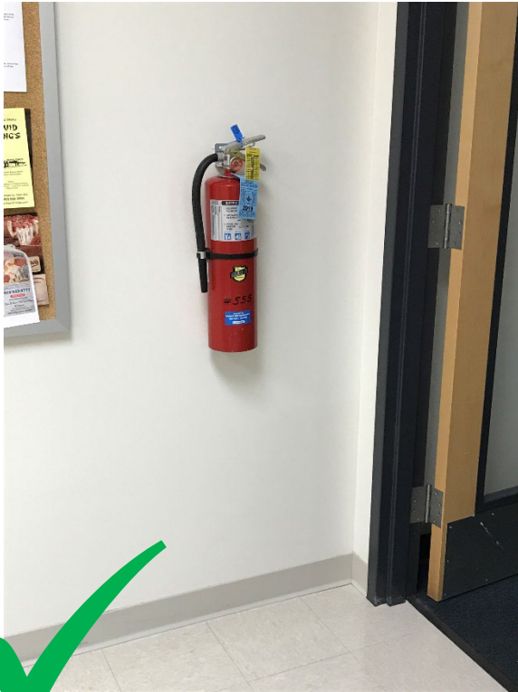
Acceptable example per MN State Fire Code 509.2
